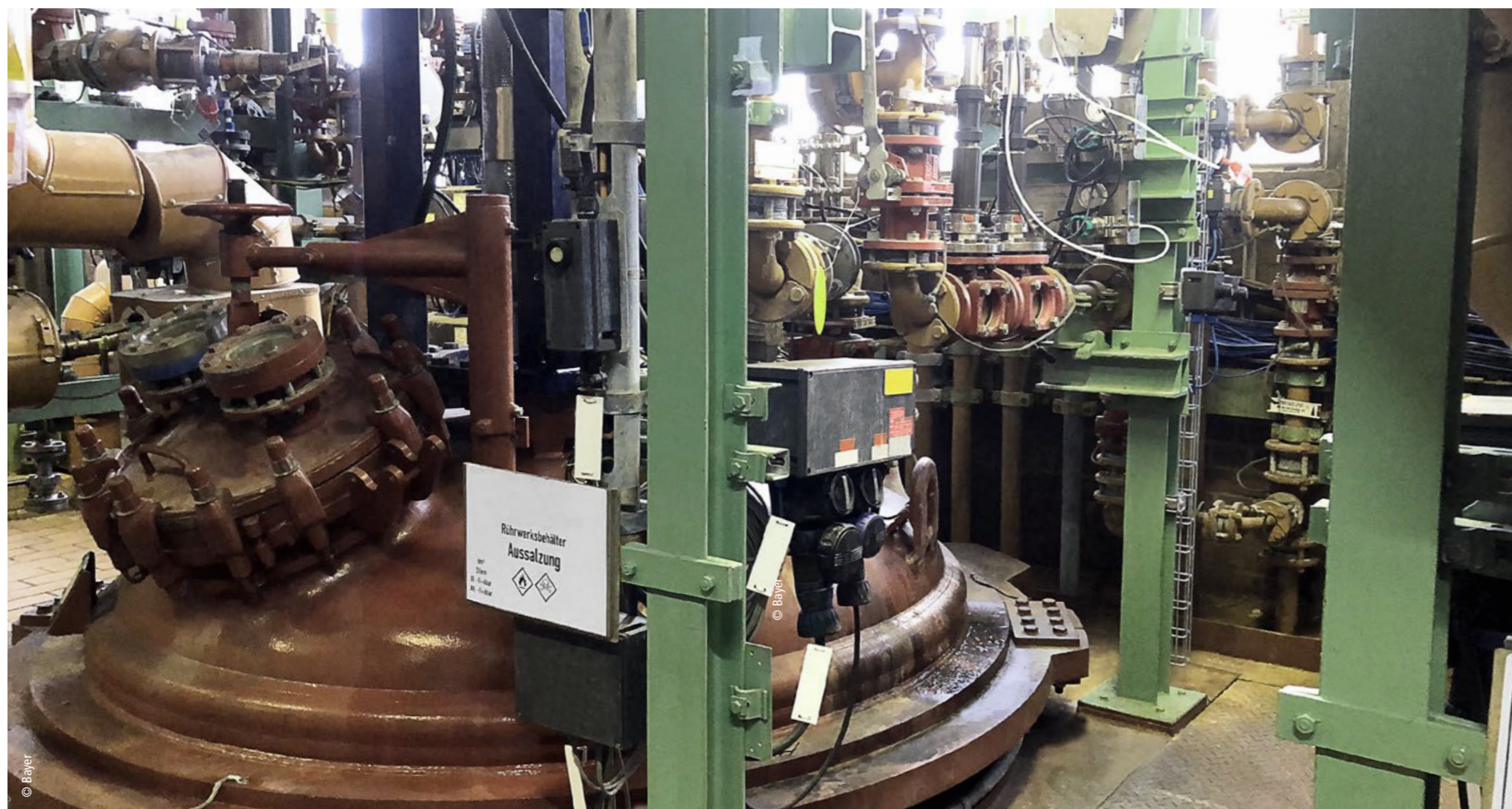
Agitator tank for desalination at Bayer's Dormagen site; here as well as in the other plants, the NOA concept can be implemented with very limited available space thanks to the highly compact solution consisting of an embedded PC and EtherCAT Terminals arranged as needed.
