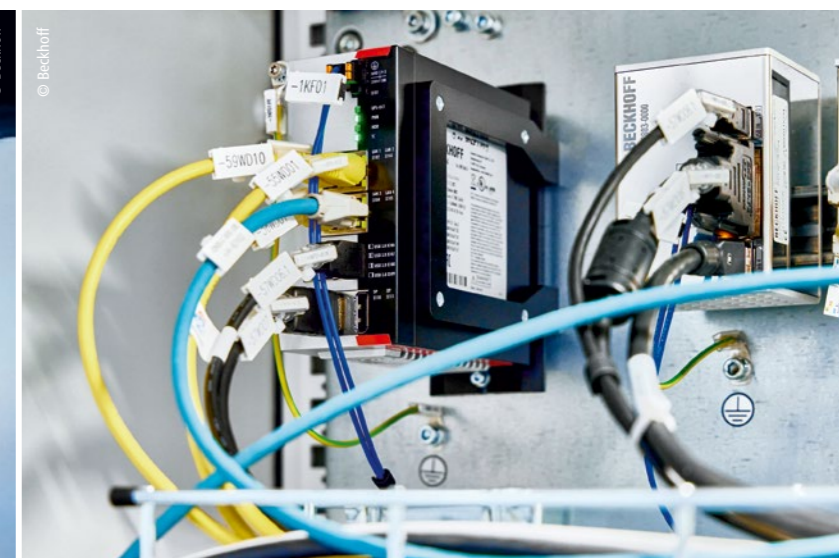
The powerful C6030 ultra-compact Industrial PC controls all machine and operating processes.
